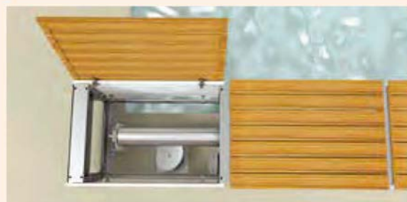
Access to the skimmers and mechanical parts
